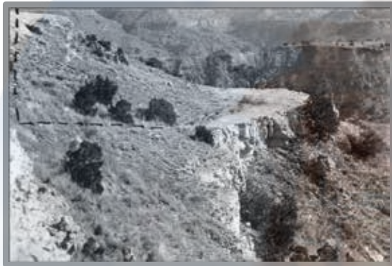
Point where the blasting took place to create the bench upon which El Coronado Lodge sits. Note the dashed lines that designate where explosives removed the soil and rock. (Image from: NARA, Denver, Co)
