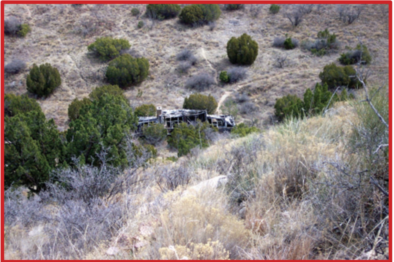
View of the CCC Bathhouse from the Park Overlook (This picture was taken several years ago. The roof has deteriorated further)
